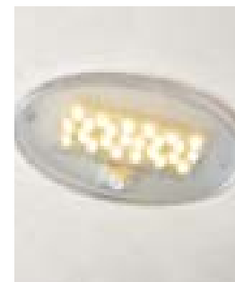
Illuminazione a LED LED lighting
